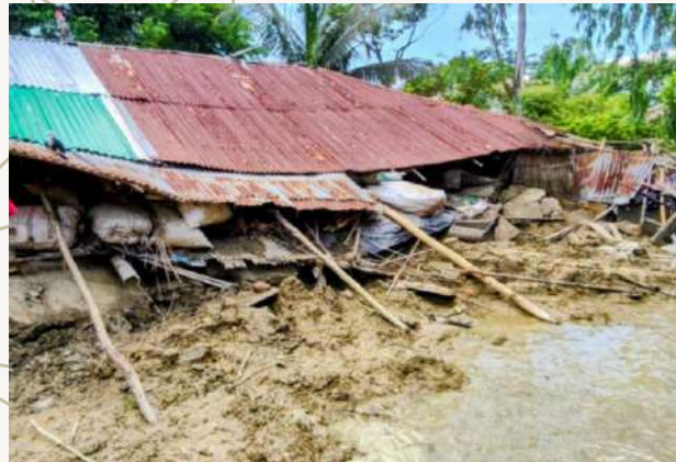
Flood damage documented for recovery planning and future preparedness.
